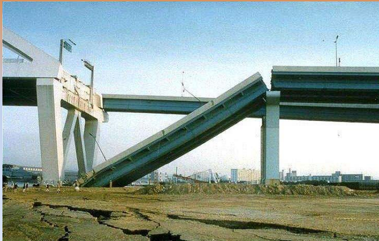
Nishinomia Bridge 1995 Kobe earthquake, Japan
